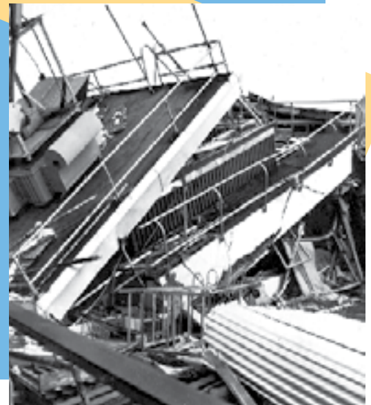
The control tower at Anchorage International Airport, collapsed by earthquake shaking. (Photograph courtesy of USGS)
