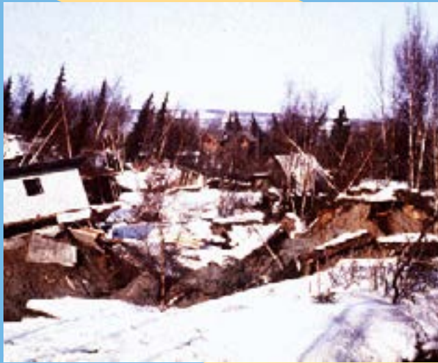
Close-up of damaged homes in Anchorage's Turnagain Heights, where homes slid into the water due to soil liquefaction and subsequent landslide. (Photograph courtesy of USGS)
