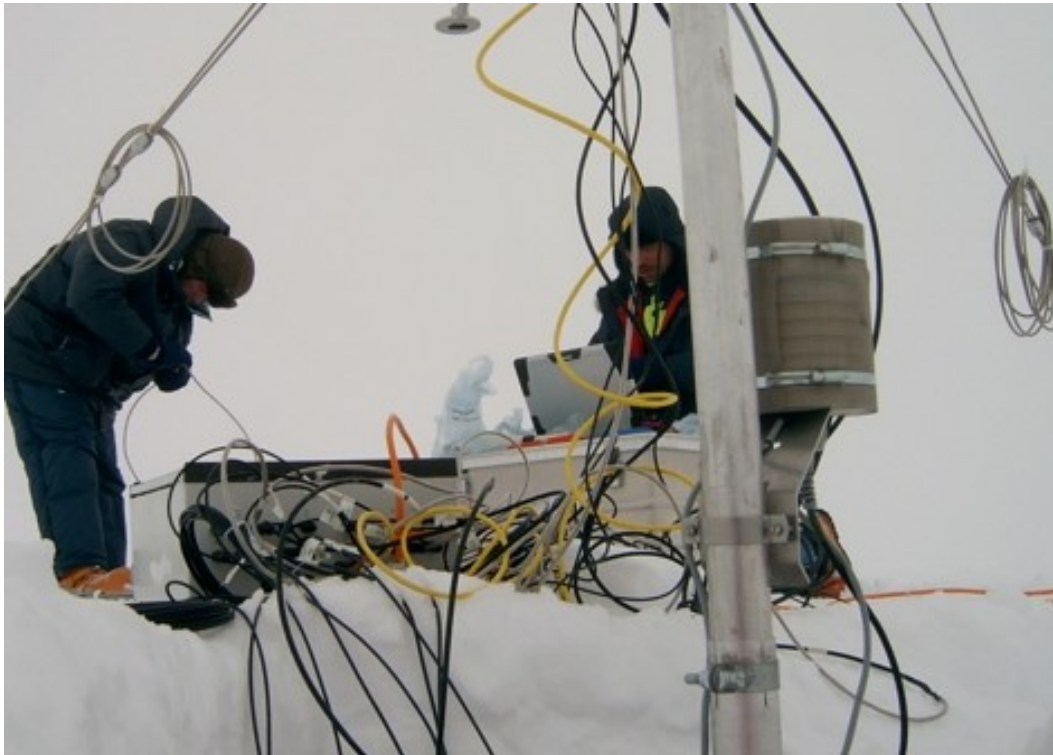
Cable spaghetti at sensor mast of full energy balance AWS during installation and configuration process (from left: Roman Finkelburg, Dieter Scherer)
